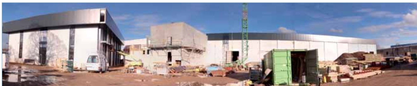
Baustellenansicht HOPPECKE F&E Center Zwickau./View of the site of the HOPPECKE R&D Centre Zwickau.
