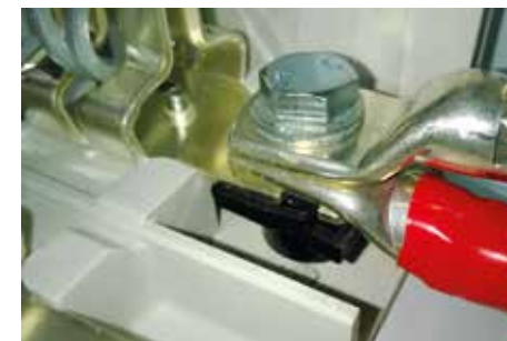
Figure 5: Cable lugs turned around to one another
