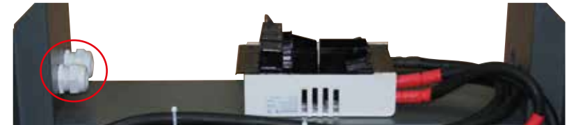
Figure 8: The upper level of the carrier with cable glands
