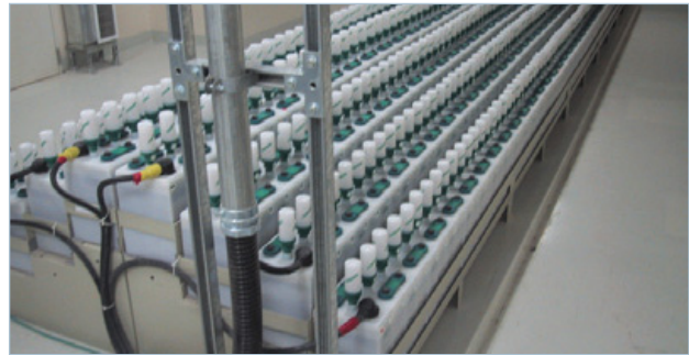
FNC® stationary battery system
